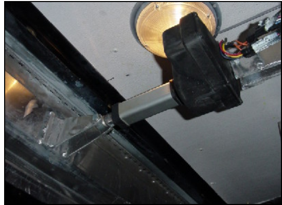
Damper with actuator – interior view
