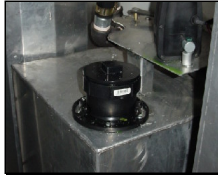
Mist Tank located inside control compartment.
